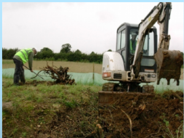
Searching for newts in the banks of a pond before draining and infilling.
