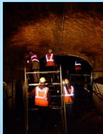
Bat Inspection survey of the railway bridge arch using a scaffolding tower
